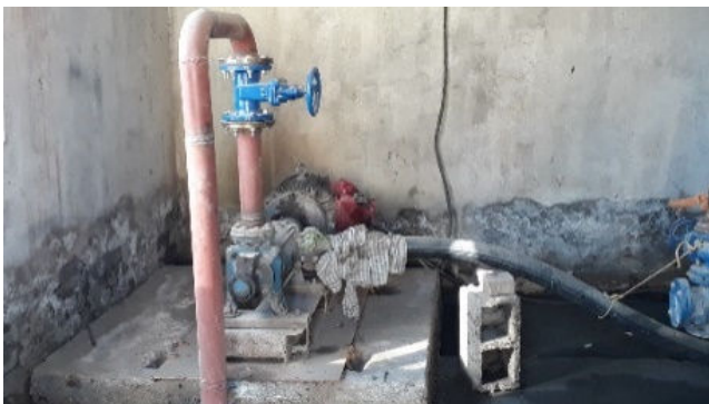
Figure 3. Pump station(after filtering) pump water for landscaping).
