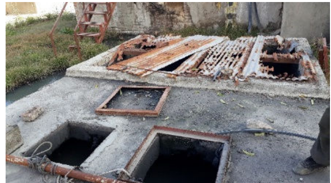
Figure 5. First storage of sewage after septic tank.
